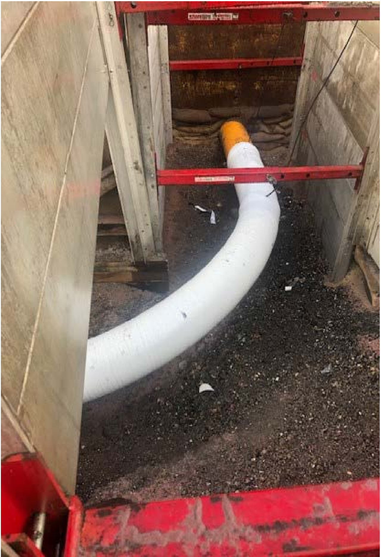
Figure 4.3 5 times diameter hot rolled induction bend installed with corrosion protection wrapping installed prior to backfill
